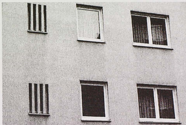
Fig. 5. Partial view of the northern façade of object 51 in Nuremberg, 17 years after refurbishment by applying a new coating in 1987. The areas between the windows, which are exposed to intense rain, are somewhat lighter, meaning that the exposure to rain did not cause the growth of algae but had a cleaning effect
