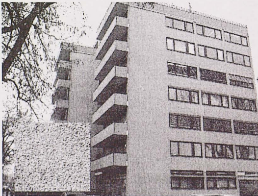
Fig. 4. Eastern and southern façade (from right to left) of object 54 in Neumarkt in December 2004, 16 years after refurbishment in 1988 by applying a new coating, close-up view of the plaster at the small window
