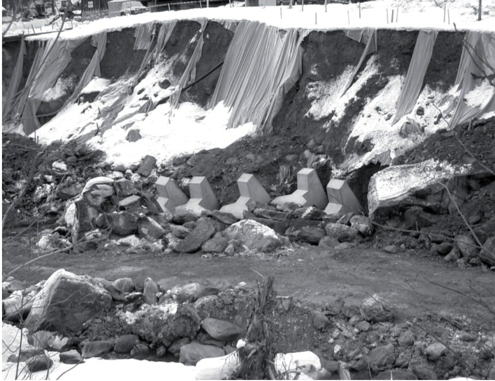
FIGURE 11. Use of heavy concrete polypode elements to increase local erosion resistance, in the steeper part of the Schwarze Lütshine river
