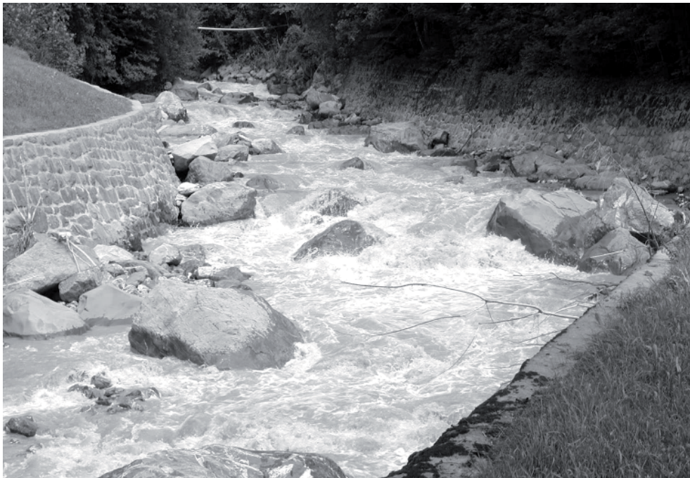
FIGURE 5. Intermediate reach downstream of the detention basin. Despite apparent stability, incision exceeding 1 to 1.5 m occurred
