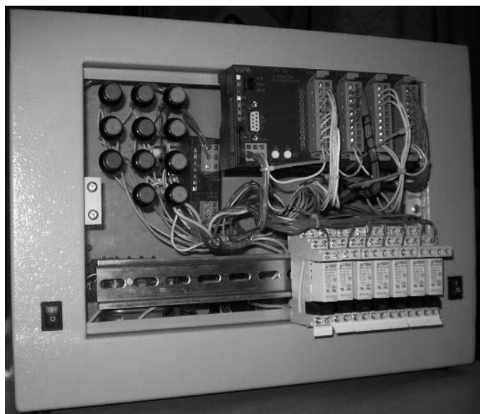
Fig.3. Robotic workcell control unit on the basis of VIPA-115 6BL02 controller
