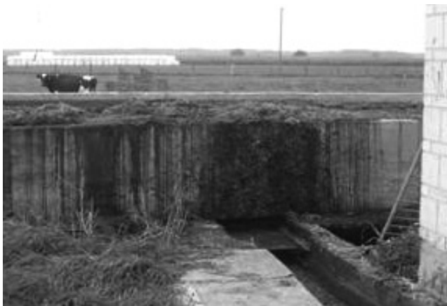
FIGURE 1. The manure board with a very small capacity (photo: K. Wiśniewski)
