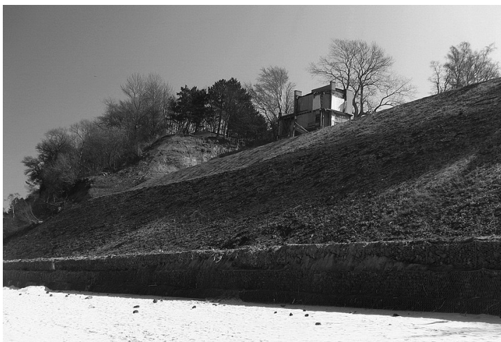
Fig. 5. Jastrzębia Góra Cliff. Landslide near Beck Villa (photo A. Marek)
