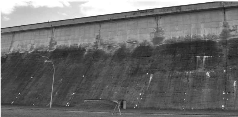
FIGURE 6a. A view of downstream wall of the water dam in Rożnów
