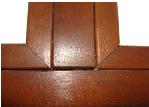
Fig. 1. Incorrectly jointed window
