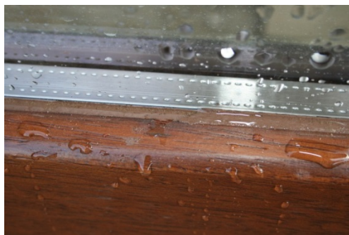
Fig. 5. Moisture condensation on the windows installed before completion of wet
