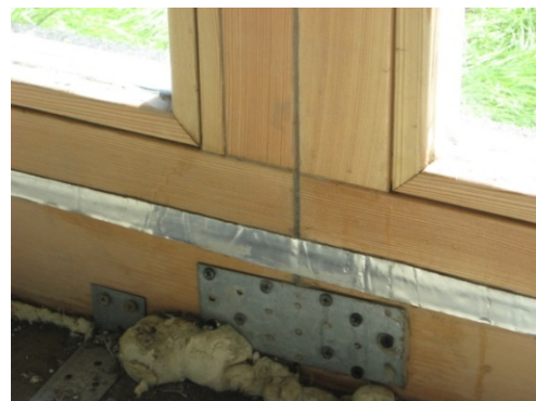
Fig. 6. Incorrect installation and sealing of adjoining windows
