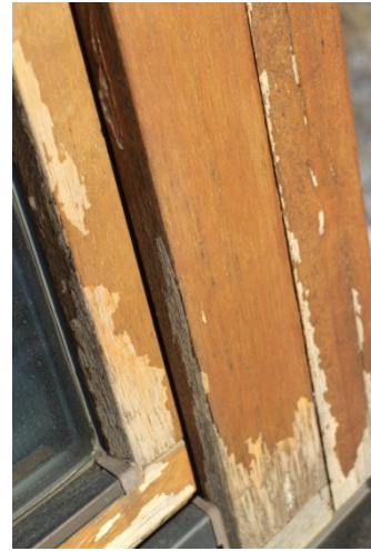
Fig. 5. Badly made protective coatings
