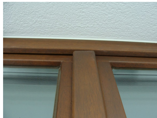
Fig. 2. Incorrect joint between the window frame and the post
