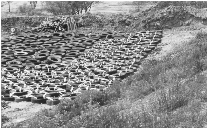
FIGURE 2. Preparation of mattresses made of used tires to reinforce of western landfill slope
