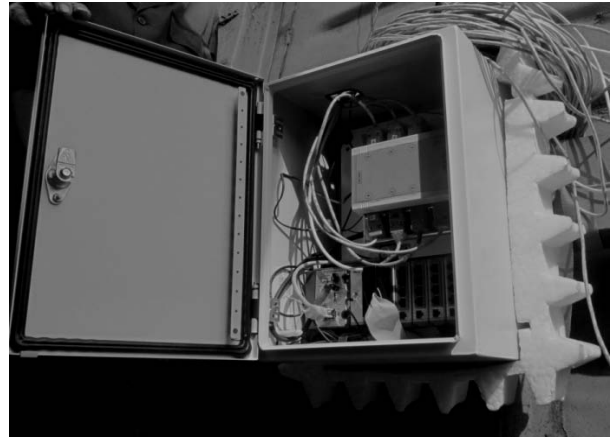
Fig. 3. A measuring equipment is in the protected corps
