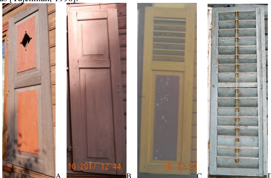
Figure 16. Double-field shutters: A- Kościuszki 19 (No.26), B- Reymonta 29 (No.65), C- Krótka 10 (No.32), D- Andriollego 35 (No.1)
