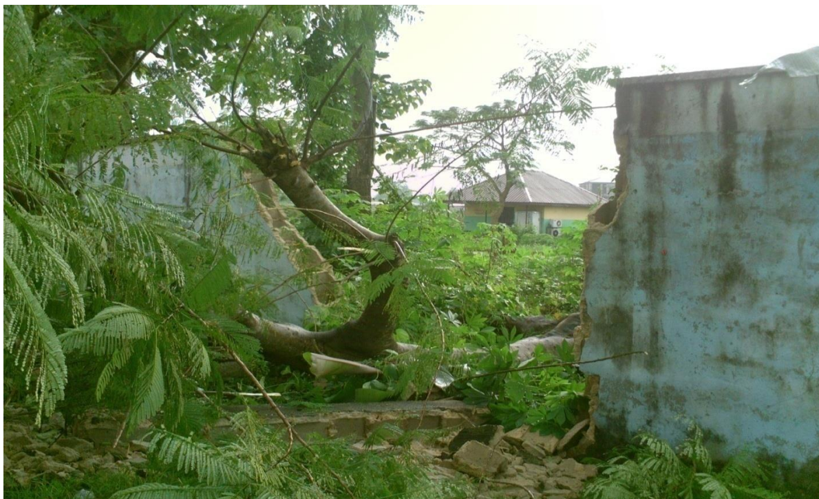
Figure 1. Pests infested Delonix regia damaging the University of Port Harcourt fence.
