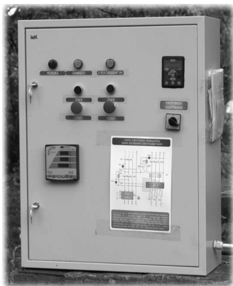
FIGURE 5. Automated system based on the motor control unit Danfoss Micro Drive
